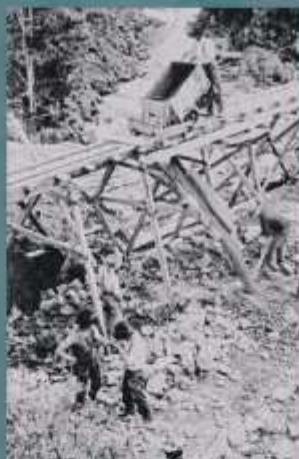
Rubble transported by train and a pulley system up hill to McLaren Falls Power Station.
