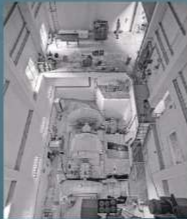
Interior of Lower Mangapapa Power Station, April 1979.
