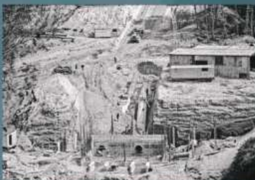
Construction of Lloyd Mandeno River Station, c. 1975. In the foreground are the four intakes of the power house and behind it are the construction offices. The concrete abutment in the background which will carry water to the 'run of river' can be seen to the right of the image. The concrete buildings are above the ground level.
