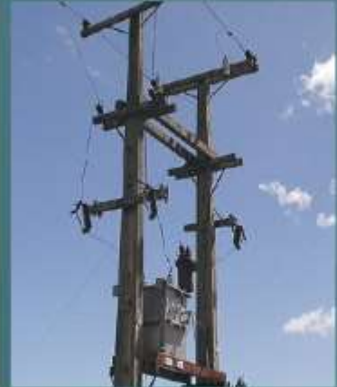
SWER 15kV transformer
