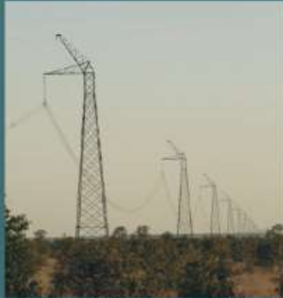
One of the two Cahora Bassa (Mozambique) high-voltage direct current (HVDC) SWER power lines as it crosses through South Africa
