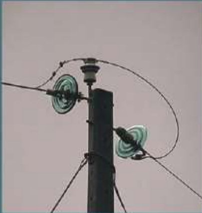
SWER Power Line
