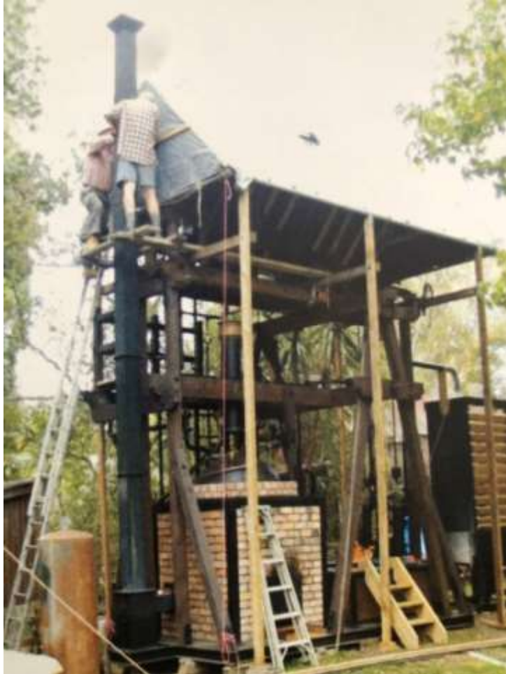
Fig 3 shows the machine during construction and provides a good perspective of the size and shape. The surrounding area is now well covered with workshops and office spaces adjacent to the machine.
