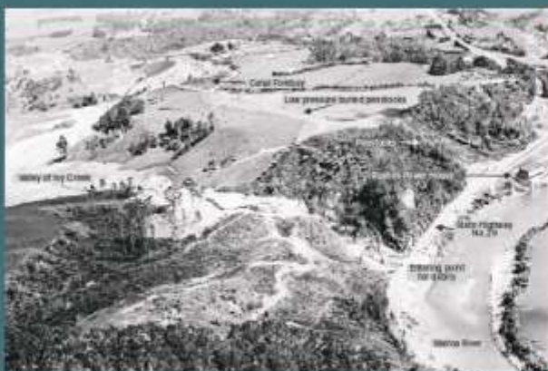
Aerial view of Ruahihi Canal after collapse on 20 September, 1981.
