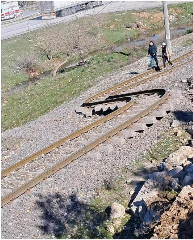
Rail displacement after Turkey earthquake.
